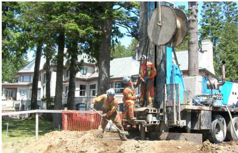
Award Winning Performance: A Sonic Drill Corporation rig drills a geothermal installation for a multi-million dollar private home in White Rock, B.C., Canada.
