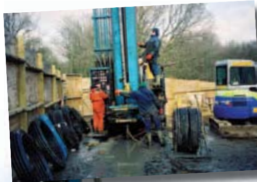
The Sonic drill-head at work. The unit can drill between three and ten times faster than conventional methods
