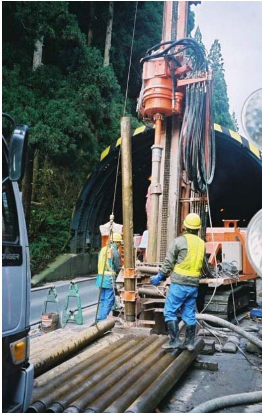
A Tone-Sonic rig, licensed and patented by the Sonic Drill Corporation, drills holes for a geothermal pavement snow-melting grid at the entrance to a highway tunnel in Akita prefecture, Japan.
