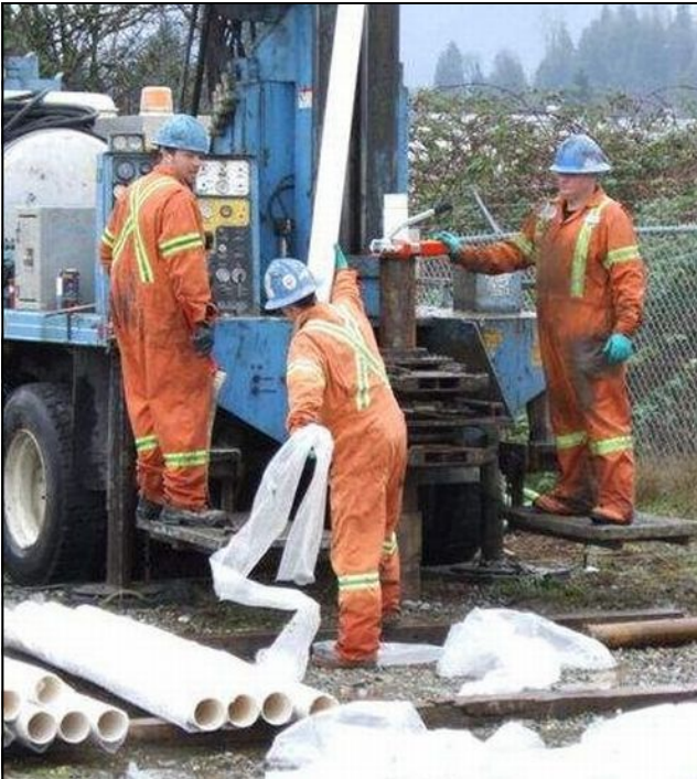
Sonic Drilling Ltd. installs a 4-inch PVC riser pipe in an observation well with a sonic drilling rig. The well is one of several observation wells to monitor the performance of a 20-inch-diameter municipal water well.
